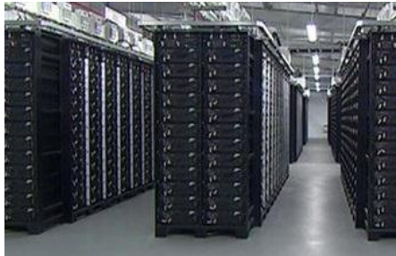
Leighton Buzzard Battery Facility
