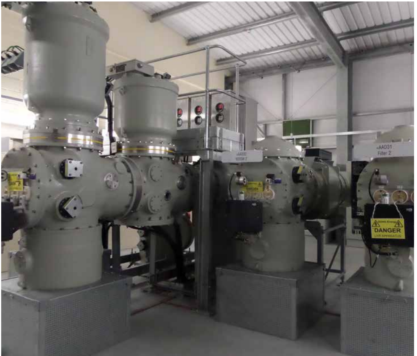
WoDS Onshore substation 155kV switchgear
