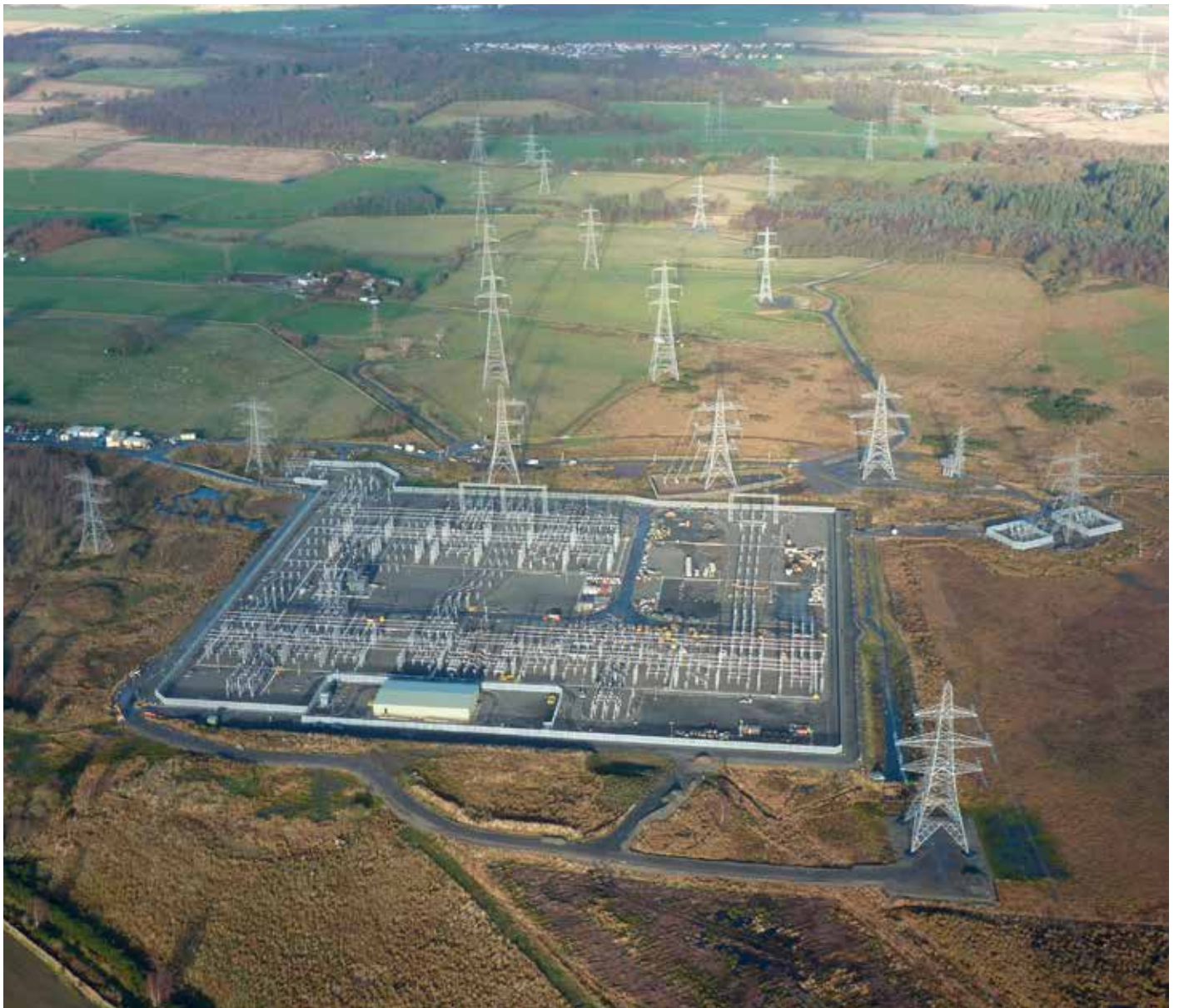
Denny North Substation
