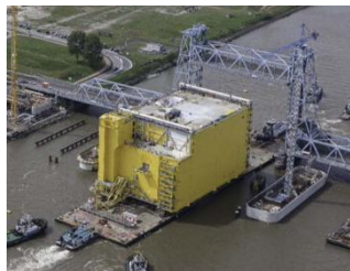
Figure E.17 DoWin Alpha HVDC topside
