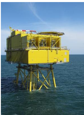
Figure E.1 BorWin1 HVDC platform, North Sea Image courtesy of ABB
