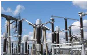
Figure E.24 Typical 132kV AIS bay
