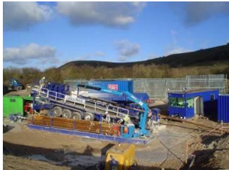
Figure E.12 HDD rig Image courtesy of Land & Marine
