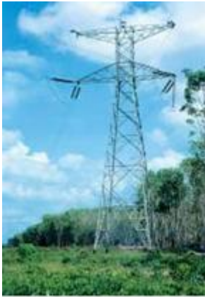
Figure E.5 Bipolar Tower 300kV Link Photo courtesy of Siemens
