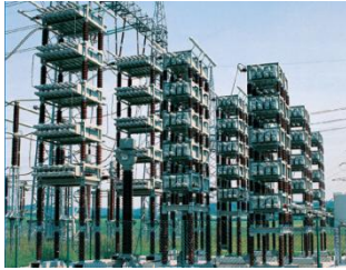
Figure E.29 Open rack capacitors Image courtesy of Areva
