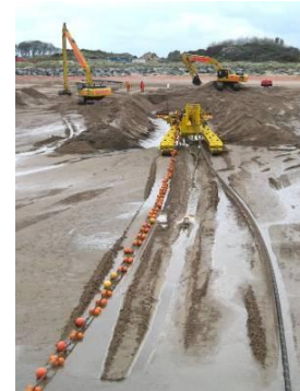
Figure E.14 Cable plough on shore Image courtesy of IHC Engineering Business
