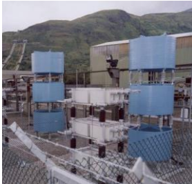
Figure E.28 Air Core Reactors (blue), image courtesy of Enspec Power
