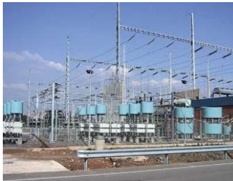
Figure E.30 Sidmed SVC, Spain, image courtesy of Alstom Grid
