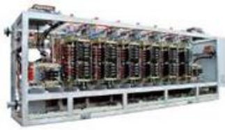
Figure E.32 32 Mvar STATCOM (building required) Image courtesy of ABB
