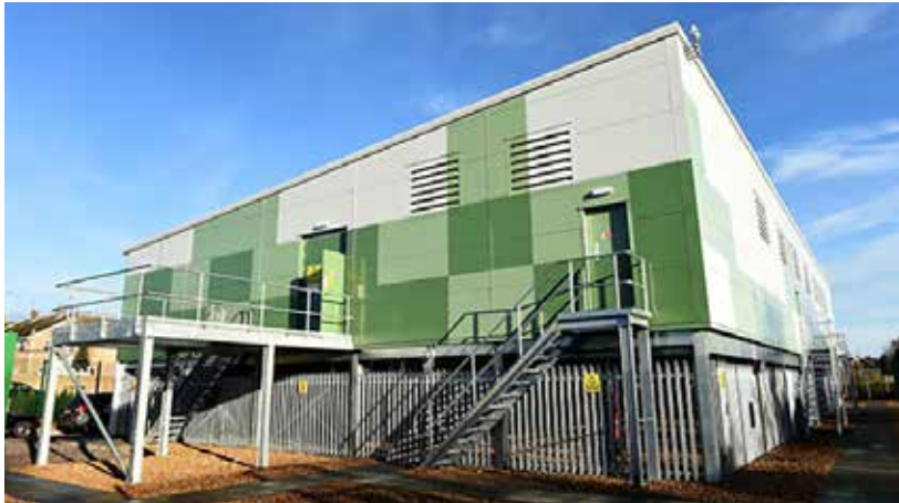
Figure 5.2: Lithium-ion battery installation
