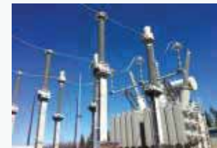
Asset Management & Monitoring
