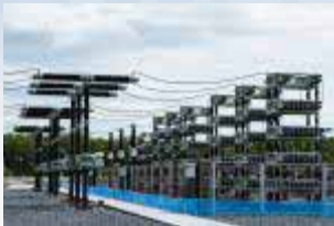
MSCDN / MSC – Capacitor Banks
