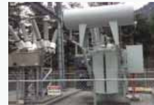
Power Transformer Energization
