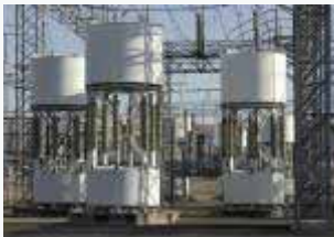
MSR – Shunt Reactors / FLT - Filters
